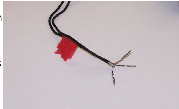
Installed Crimp Pins
